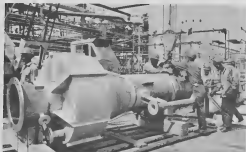
While still on its pallet, the 14-ft. tall smokeless tip is secured for lift-off.
